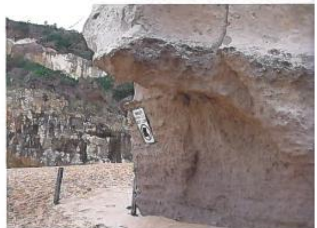
Figure 2 Cliff undercutting and weakening
